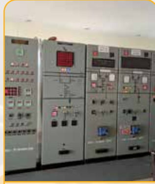
Electrical Control Panel
