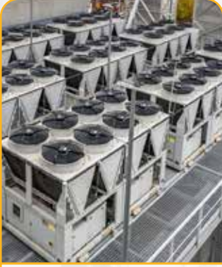
Air Cold Chiller
