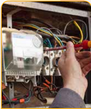
Building Electric Wiring
